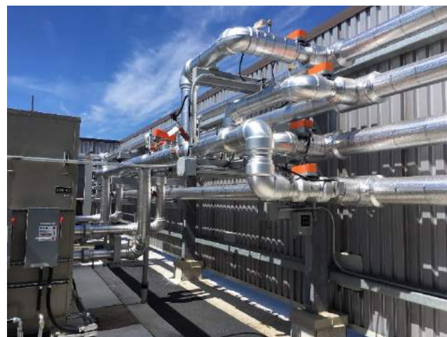
LEVEL 9 WATER / AIR HEAT PUMPS
