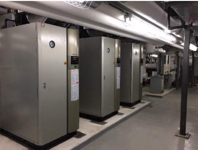
LEVEL 9 STEAM BOILERS
