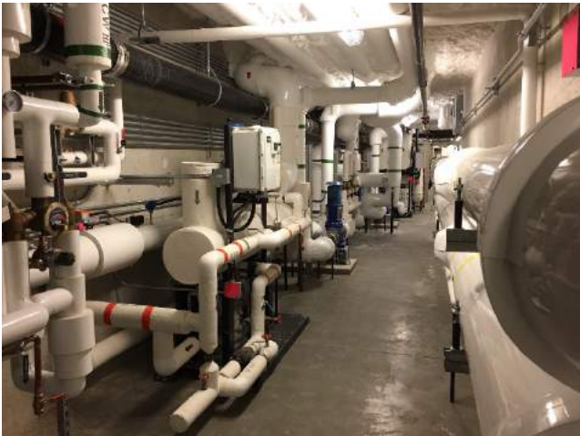
LEVEL 0 MECH ROOM
