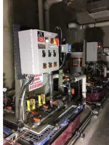
LEVEL 0 CHLORINATION SKIDS
