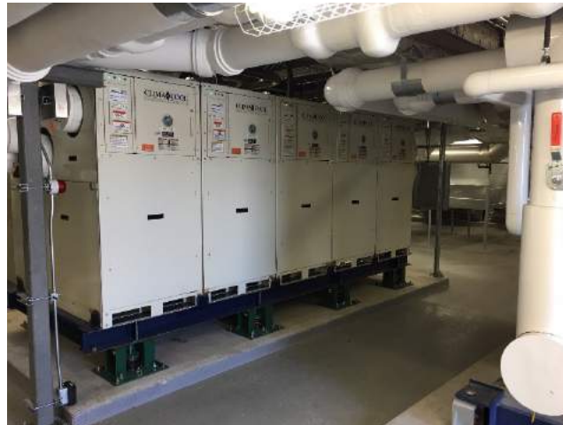
LEVEL 9 HRU-1 HEAT RECOVERY UNIT
