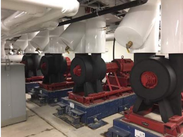
LEVEL 9 CHILLED WATER PUMPS
