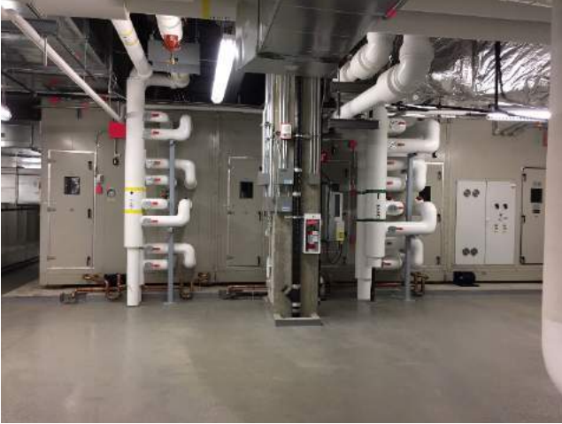
LEVEL 5 AHU UNIT
