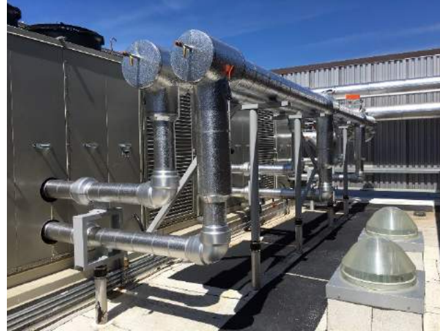
LEVEL 9 WATER / AIR HEAT PUMPS
