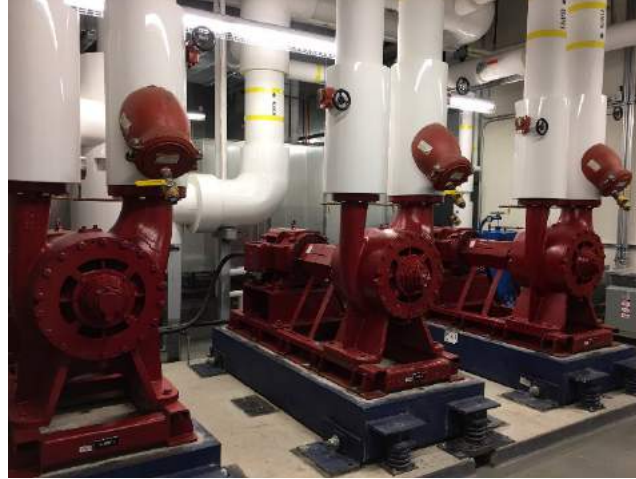
LEVEL 5 MAIN HW PUMPS
